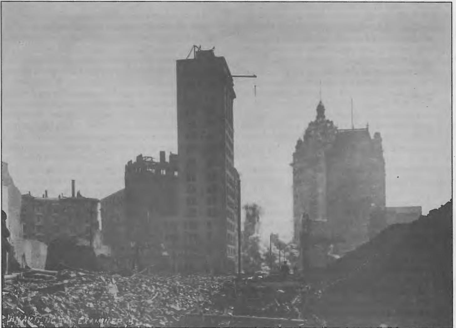
Figure 13: Dynamiting the Hearst Examiner building on the morning of April 18, 1906. View from Kearney Street south towards Market. Note that the Call, or Claus Spreckels, Building, the tallest early Skyscraper west of the Mississippi, at center right is just beginning to catch fire. The Call Building caught fire through gaping windows broken by the earthquake, sparks were drawn up its elevator shaft, and it burned from the top down. J. Stoddard photo, courtesy of the California Historical Society/Bancroft Library of the University of California, Berkeley.
