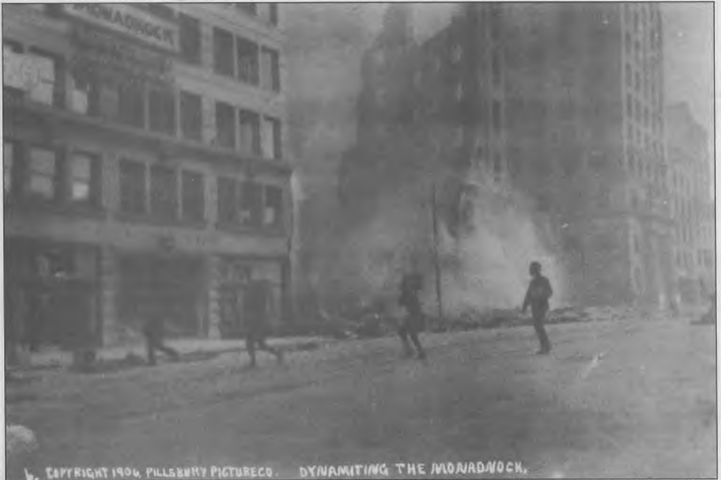
Figure 7: Two regular U.S. Army soldiers, part of a four-man fire-fighting demolition squad, running across Market Street with boxes of stick dynamite on their shoulders on the morning of April 18, 1906. The explosives will be placed within the ground floor of the still-unfinished Monadnock Building, one of the most modern in the city. To the right of the Monadnock are the smoking ruins of the Hearst Examiner Building, just dynamited. To its right are the lower floors of the 18-story Call Building, whose upper stories were aflame. The dynamiting of the Monadnock was unsuccessful; the explosives blew out the front wall of the building, but left its steel girder frame unharmed. Photo by the Pillsbury Picture Co., courtesy of the California Historical Society.
